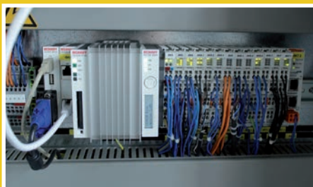
03 Controller with I/O
